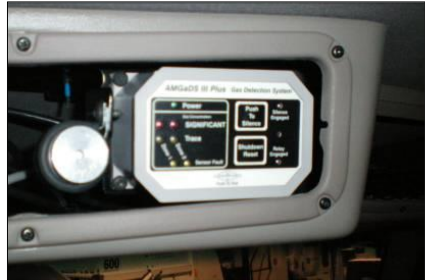
In overhead console
